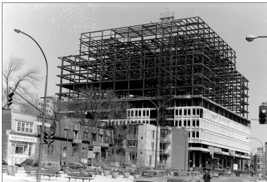
Figure 2. Hall Building under construction, ca 1965. View from Guy and de Maisonneuve (then Saint-Luc/Burnside). P184-02-0, Concordia Archives.
